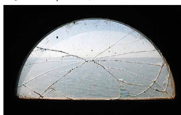
A broken window stands as a testament to the badly needed repairs.
